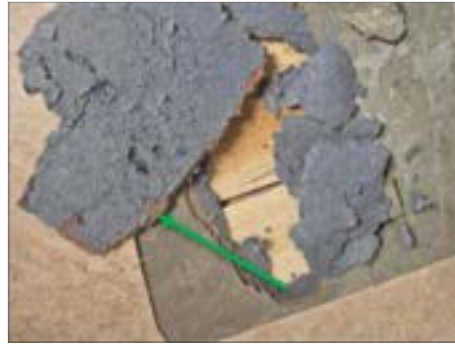
✓ 10003:1 + 10027:1 + 10021. Under dold linoleum. Brunt lim. Ej asbest.
