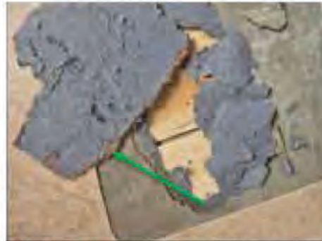
✓ 10003:1 + 10027:1 + 10021. Under dold linoleum. Brunt lim. Ej asbest.
