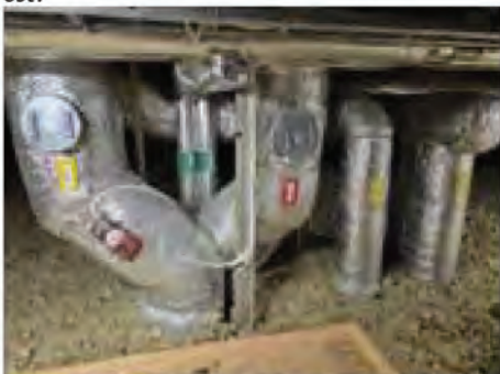
By 111 plan 13. Nyare ventilationsinstallation.
