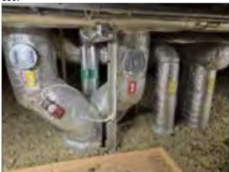
By 111 plan 13. Nyare ventilationsinstallation.
