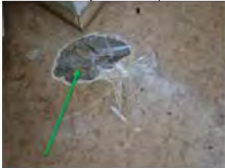
✓ 11003:2 Svartlim + underlagspapp under linoleum. Ej asbest.
